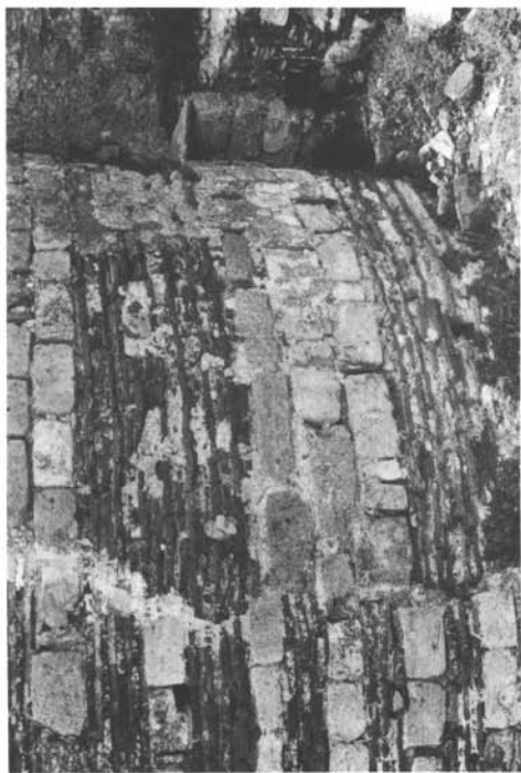
10 Enez. East facade, main apse. Detail of construction technique: recessed brick to right: later repairs to left
